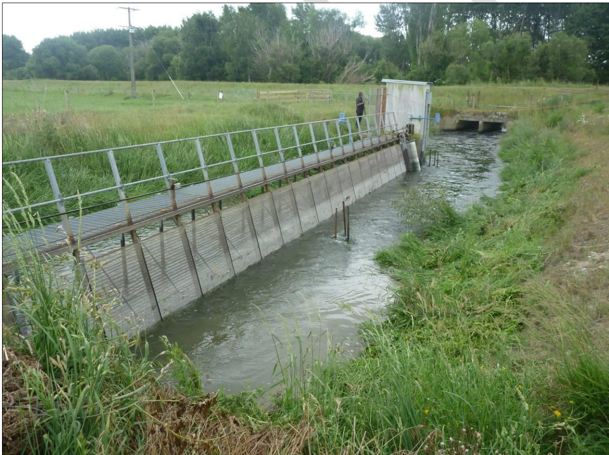
Figure 1. The Levels Plain irrigation screen on 7 December 2010. The DIDSON is positioned halfway along the length of the screen, supported by warratahs. The upstream control gate is positioned upstream of the bridge. Photo by Sjaan Bowie.
